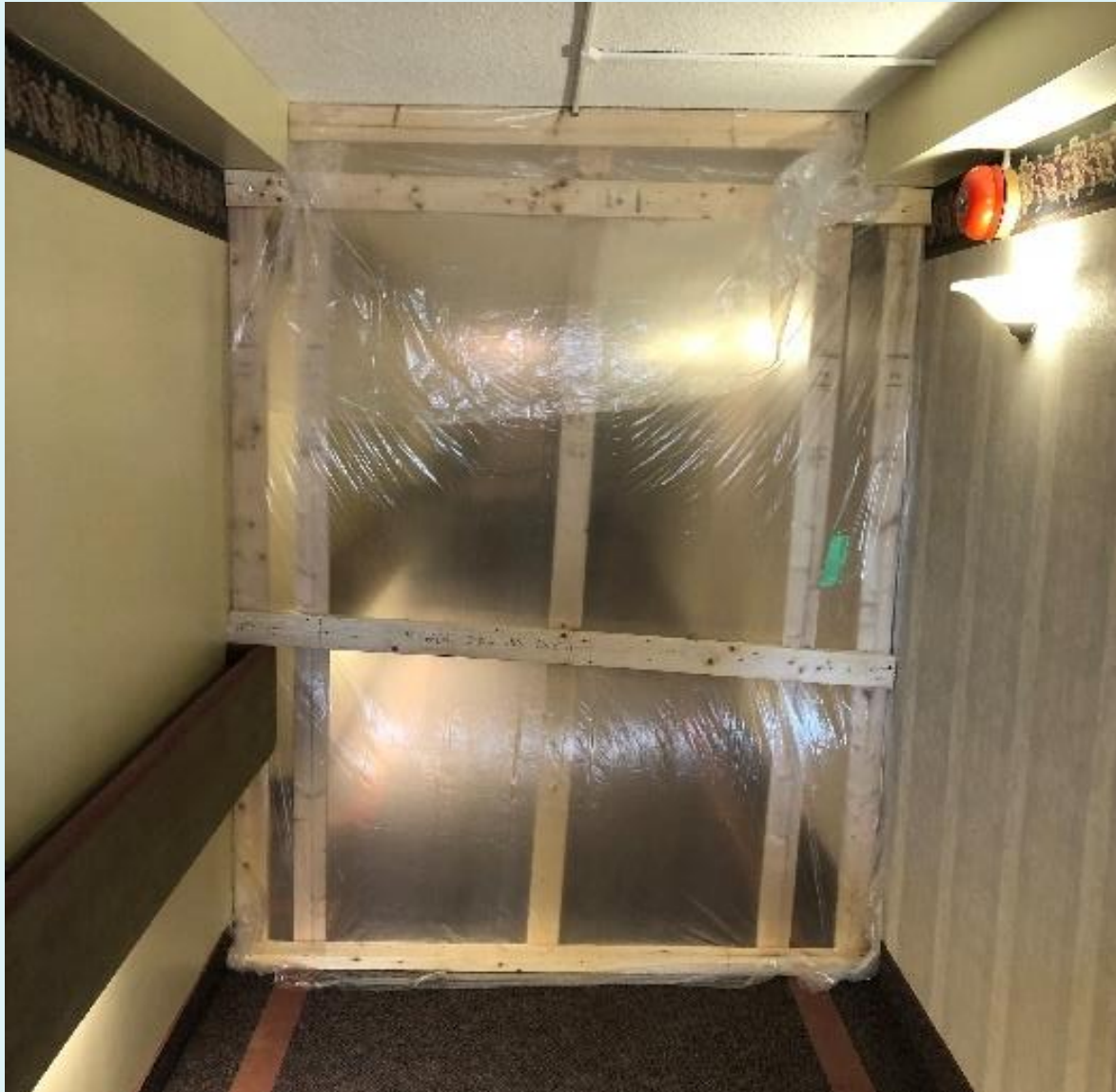
Figure 9: example of a temporary partition to separate two areas of the building during testing
